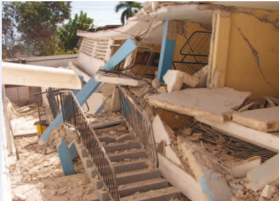
Above: The destruction: one of the schools that collapsed during the earthquake Below: The reconstruction begins: rebuilding St Martin's School
