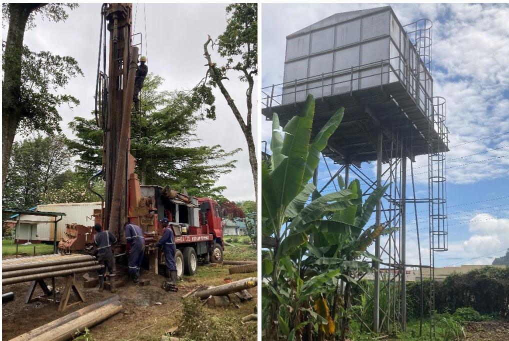
Sinking the borehole & new water tower. Now waiting for the electric pump to start using the water
