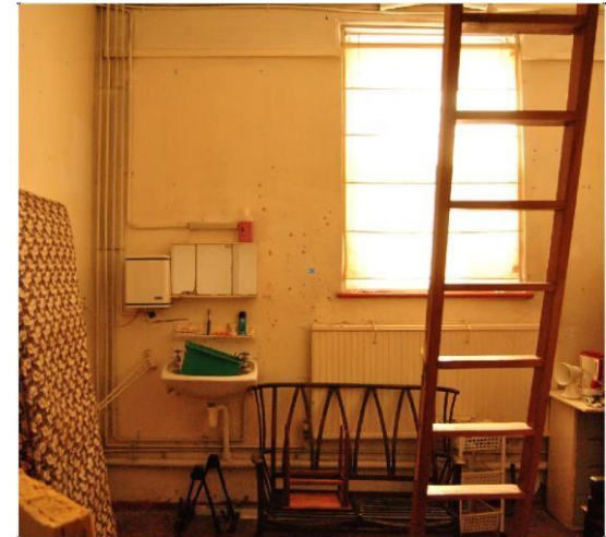
Interior: Unsafe Student Accommodation abandoned since 2008
