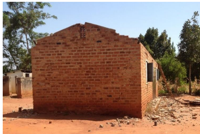
Burnt manse in need of renovation for new MCU minister
