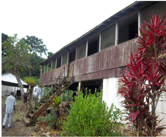
Church manse still in use but in a precarious state
