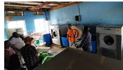
Laundry. All machines not working.
