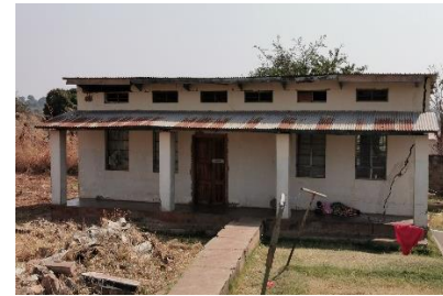
Laundry room falling down.
