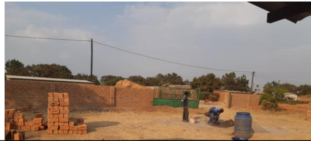
Jane oversaw the completion of the new wall around play4all. The builders used the hand moulded mud bricks common in Zambia
