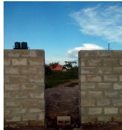
The new wall, looking through the pedestrian access towards the food production classrooms
