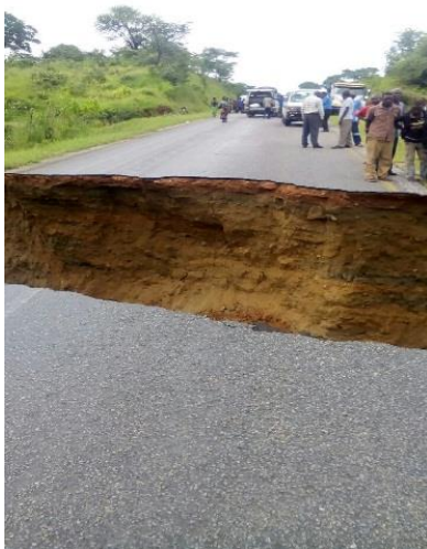
The road to lake Kariba damaged by flood water.
