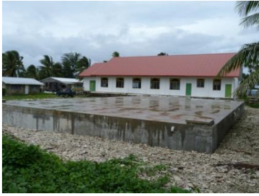
The new, 700,000-litre water tank at Lofeagai
