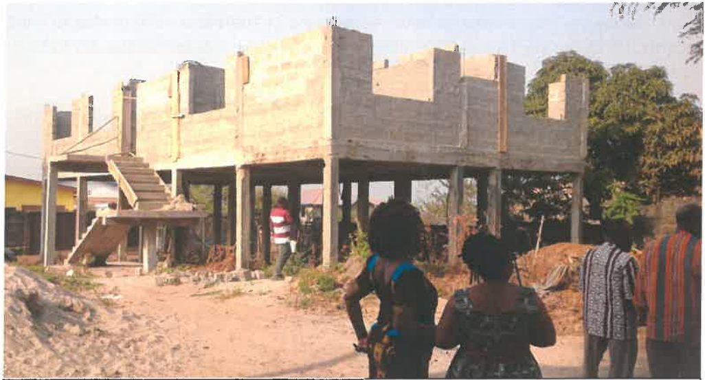
The construction of a new Community centre for PLHIV funded by Isle of Man MC
